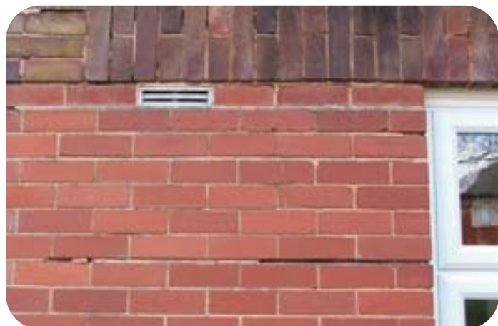
e.g. an example of failing cavity wall ties
