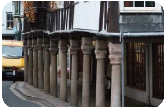
e.g. an example of foundation movement
